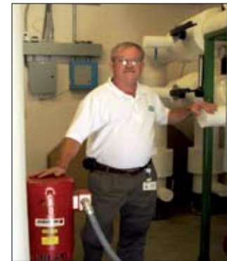
Jim Barr, Daviess County Public Schools' energy manager, stands in a room that houses Southern Oaks Elementary's geothermal pumps. The school earned a 92 percent ranking from Energy STAR, a government-backed program that promotes conservation.
