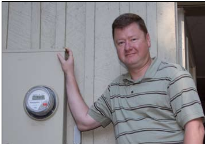
Billy Boyle, a Kenergy member-owner who lives in Owensboro's Bon Harbor subdivision, likes the convenience of his automated meter. Boyle is one of about 1,100 Kenergy customers on a pilot program titled Automated Meter Infrastructure.
